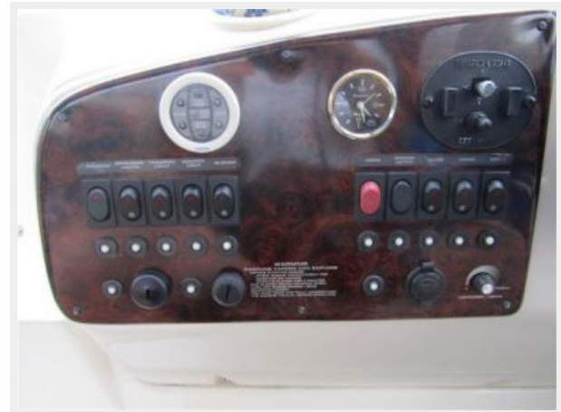
33' Rinker 3300 Fiesta Vee Helm electrical panel
