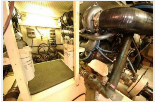
Engine room photo 3
