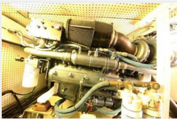
Engine room photo 4
