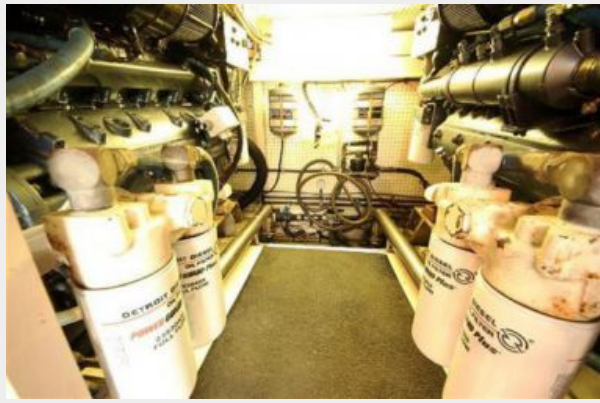
Engine room photo 2
