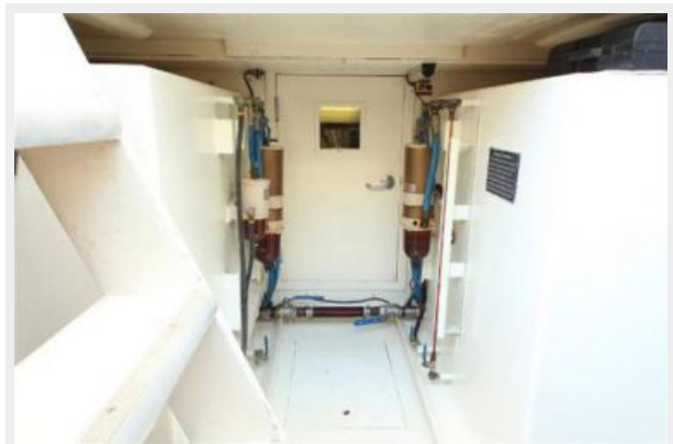
Fuel Tanks with filters and sight glass
