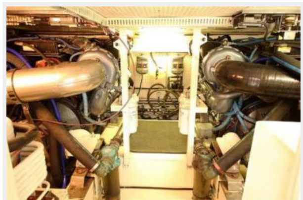
Engine room photo 1
