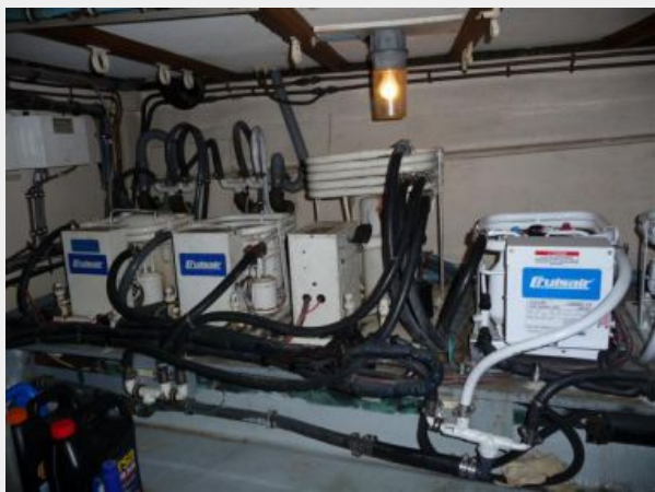
Gen/Room AC Units
