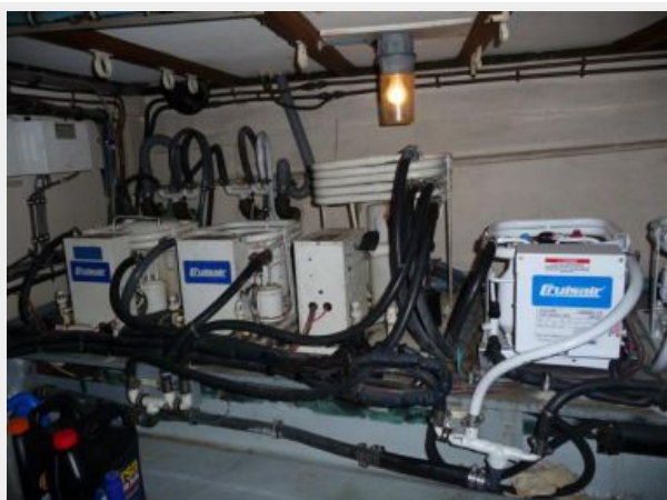
Gen/Room AC Units
