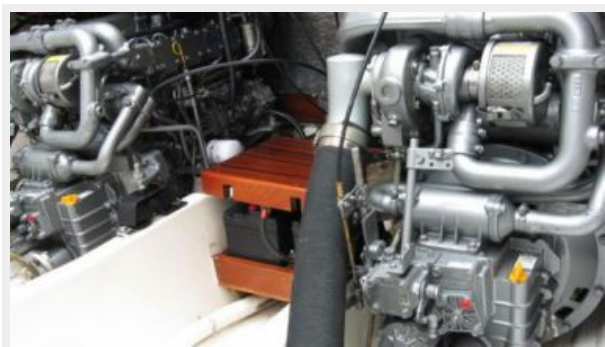
Very clean engine room
