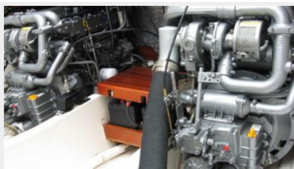
Very clean engine room
