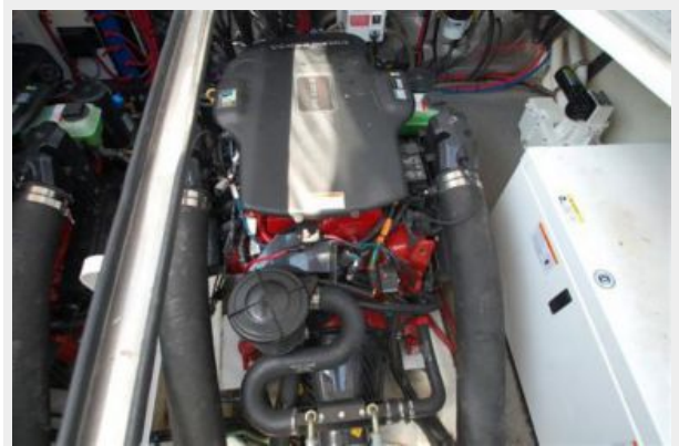
Starboard Engine & Genset
