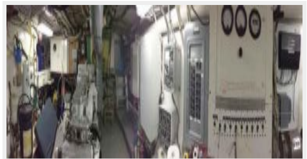
Panoram Engine Room
