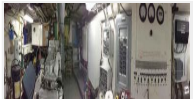
Panoram Engine Room
