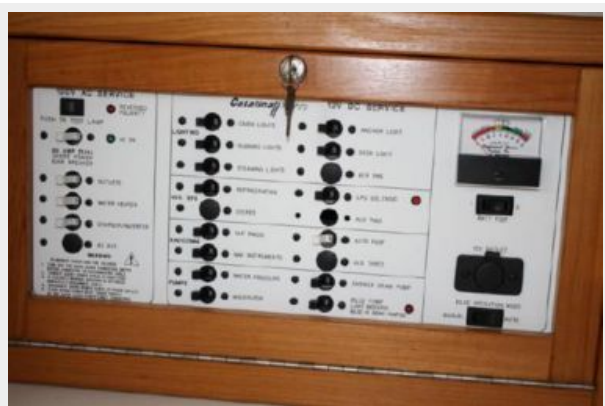
Electric breaker panel
