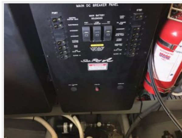
Main DC breaker panel
