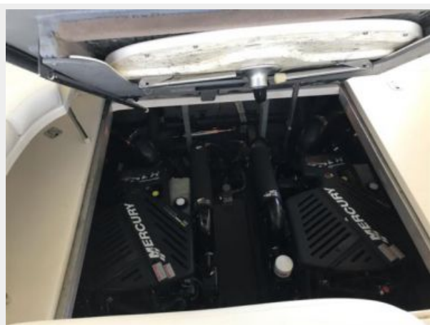
Access to the engine room
